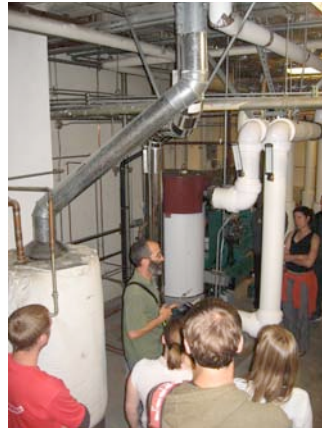
Richard Engel discusses boiler efficiency.
