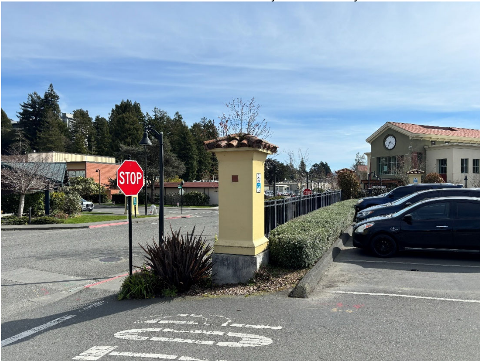
Photograph 3 – Parking Lot G11 retaining wall column and south lot exit – red paint (typical) contains lead – view looking south
