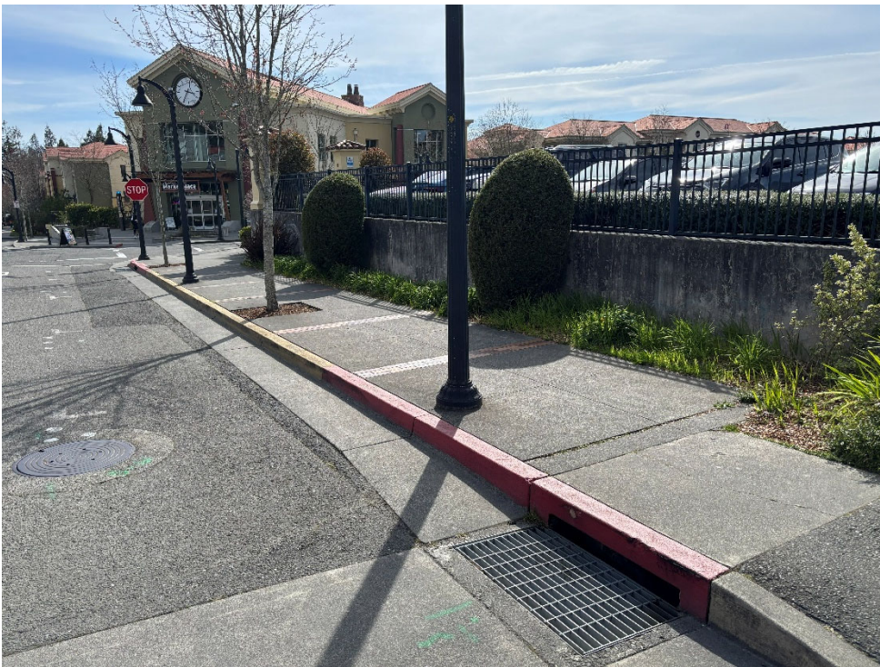
Photograph 2 – Parking Lot G11 retaining wall and Rossow Street sidewalk – red paint (typical) contains lead – view looking southwest
