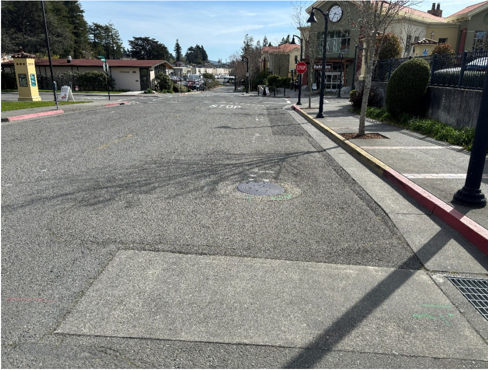
Photograph 1 – Rossow Street – red paint (typical) contains lead – view looking south
