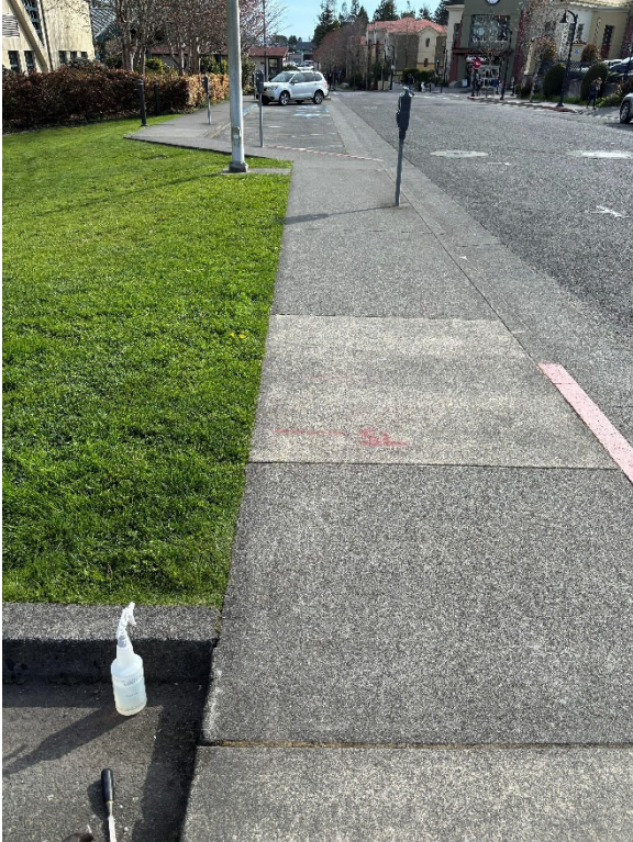
Photograph 5 – Rossow Street east sidewalk – red paint (typical) contains lead – view looking south
